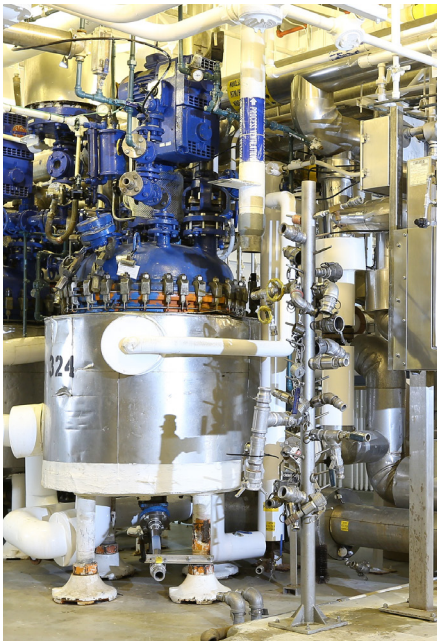
400L Reactor Train
