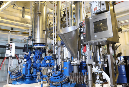
800L Reactor Train
