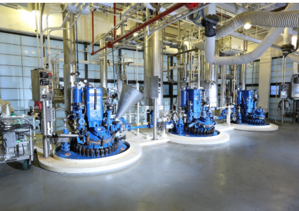
4000L Reactor Train
